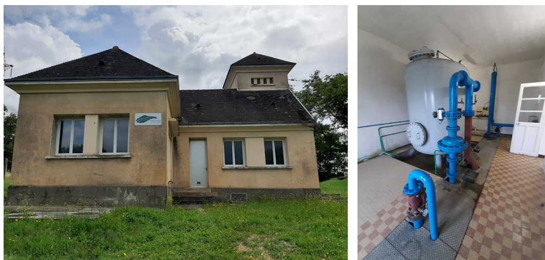
Figure 5 : Station de production Sacierges 1
